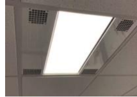
Ceiling Filter Unit
